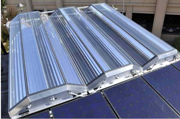
Fig. 1: Detailed view of the CPV-T ANU-Chromasun MCT system installed alongside a conventional PV system on the same mounting support.
